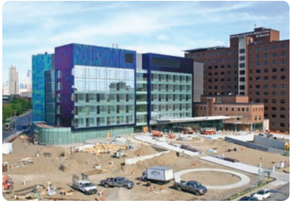
The new University of Minnesota Amplatz Children's Hospital facility will open in late March 2011.
